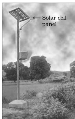
Figure 14.7 A solar cell panel
